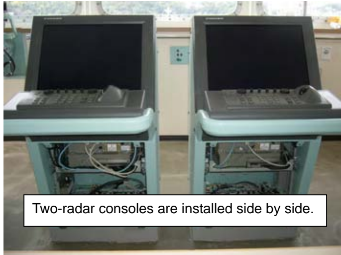
Fig. 1.4.1 Installation of two-radar consoles
