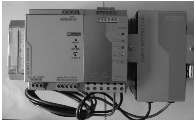
Fig. 8. View of UPS6
