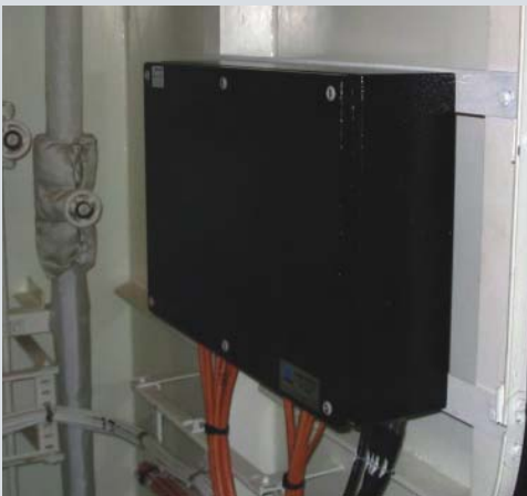
Data Acquisition Unit (DAU)
