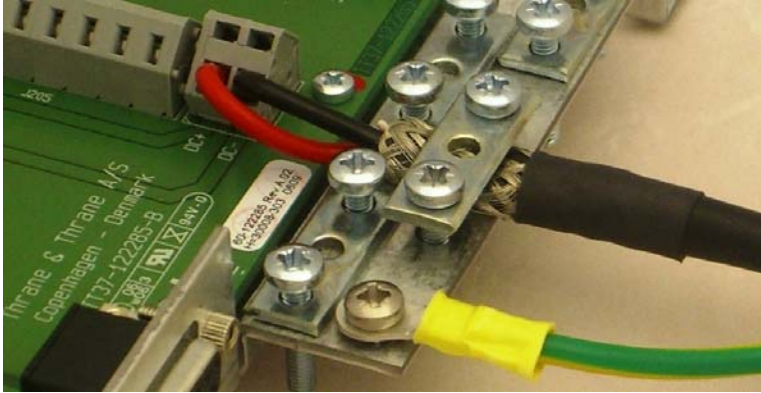
Figure 17 Power cable connections.
